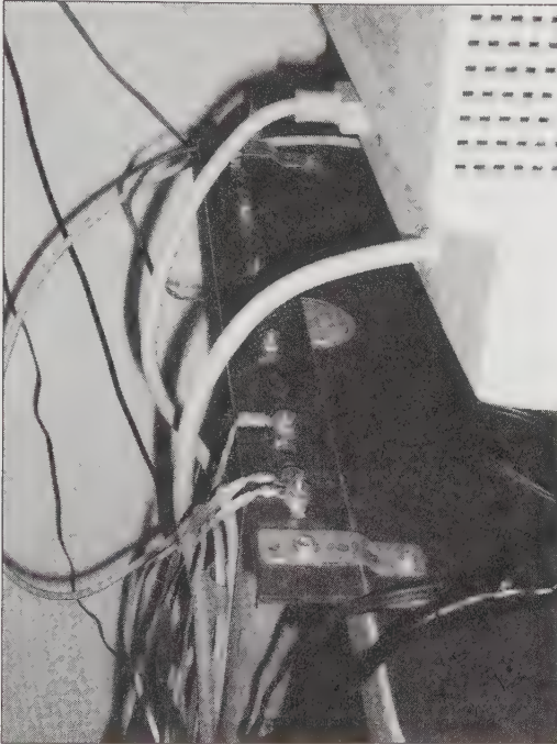
Figure 13-10: A copper bonding bus.
