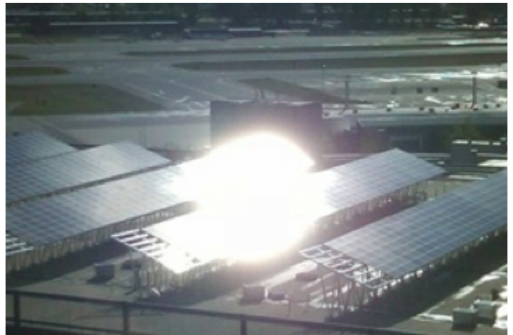
Federal funds built these solar panels which are now blinding pilots.
